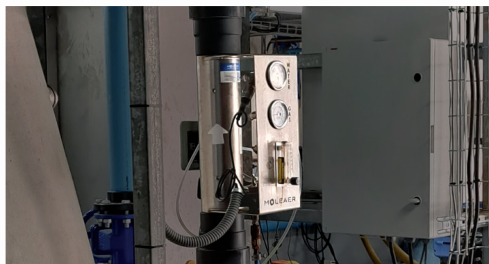
Figure 2. Integration of the Trinity L1 nanobubble generator into the existing system, replacing the traditional oxygenation cone.
