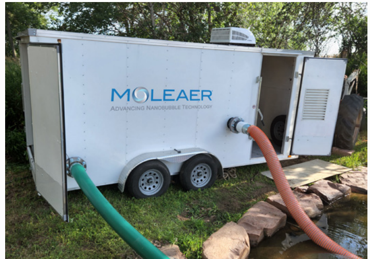
Figure 2: A 1000 GPM nanobubble generator with both oxygen and ozone generators were installed on the lake.
