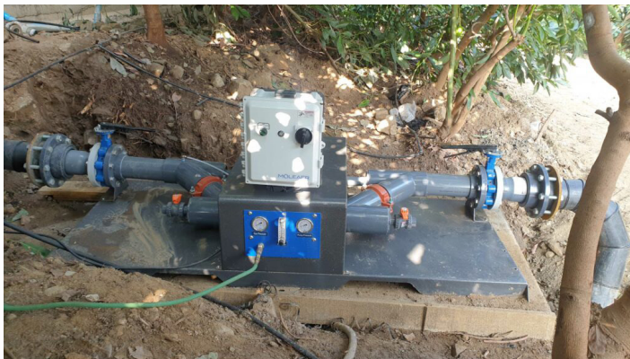
Moleaer's Nexus™ nanobubble generator was installed in-line with existing irrigation systems to supersaturate irrigation water through drip irrigation lines.
