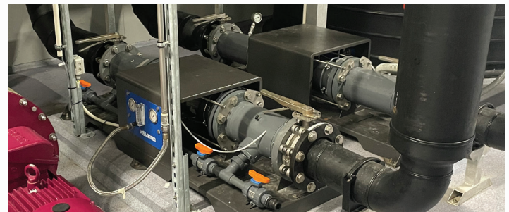
Figure 1. Installation of Moleaer Trinity L2 nanobubble generators for main oxygenation at Lødingen Fisk RAS facility. The L2 Trinity units have a liquid flow capacity of 230 m 3 /hr (1000 gallons per minute) each and an Oxygen injection rate of 5 to 50 SLPM. They were installed recirculating the water from the biofilter into the header tanks.
