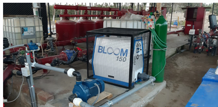
Moleaer's 25 GPM nanobubble generator was installed next to an irrigation water tank for continuous water treatment during the testing.
